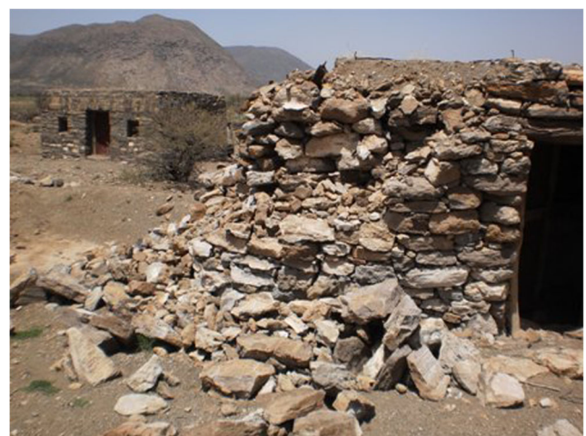
Fig. 5 Building damaged by the 31 March 2011 earthquake. Better constructed walls, as seen in the background, sustained only cracking
