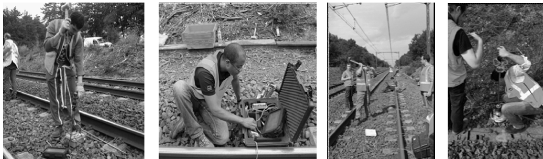
Figure 7: Test campaign carried out on the Vierzon site, (a) Panda 3®, (b) geo-endoscopic tests, (c) MASW and (d) dynamic load plate test [13].
